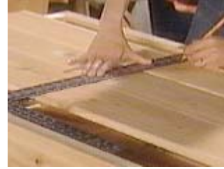
Use a straight edge to mark for the deck screws; two screws an inch from either edge of the board
