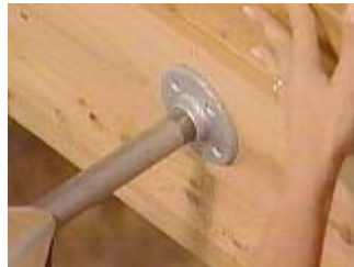
Galvanized flange and pipe attached to the tray.
