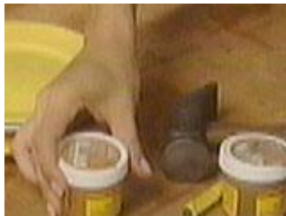
Fill the nail holes with oil based putty mixed to the correct colour
