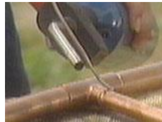
When it's hot enough, the solder melts and flows into the joint
