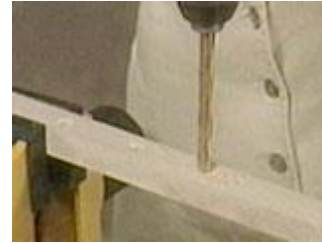
Use a counter sink bit or larger bit to cut a space for the screw head
