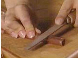
To drill the holes, first file a little flat spot on the pipe
