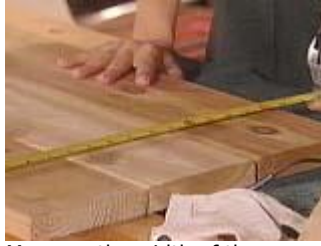
Measure the width of the bottom boards and cut a side board to fit.
