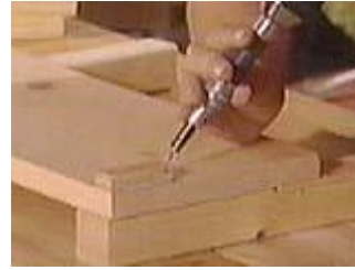
Use the jig to locate the position of the screw for drilling.
