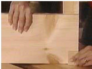
Make a new jig for the front so that the screws go into the corner posts.
